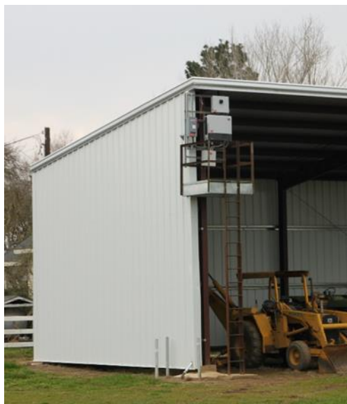
Figure 24: Elevated Electric Service and Equipment
