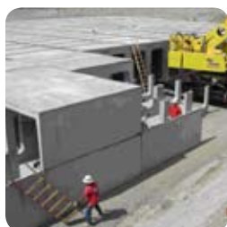
Subsurface infiltration basin in Rancho Mirage, CA. Photo courtesy of RGA Landscape Architects.
