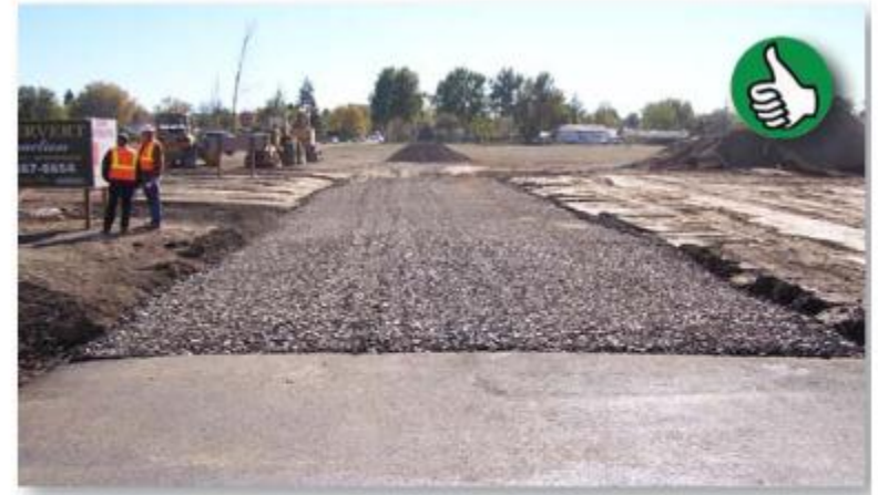
An excellent example of a properly installed construction entrance. (Source: Asotin County)
