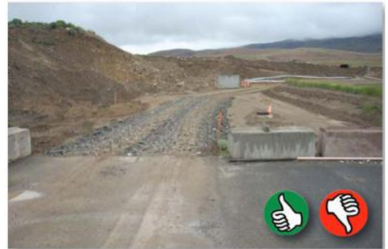
Good installation of a construction entrance, but sediment is still being tracked off-site. Add more rock or make entrance longer. (Source: Douglas County)
