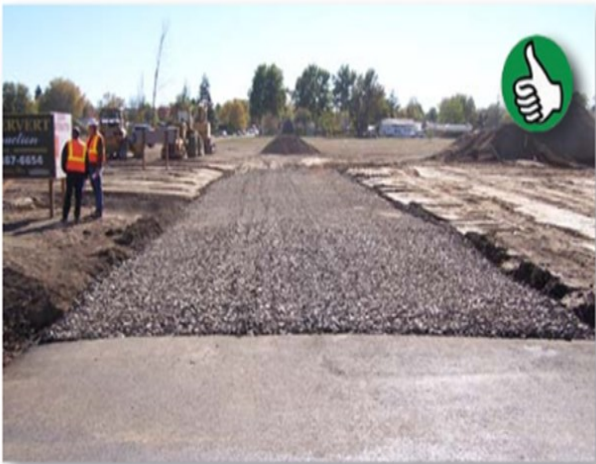
An excellent example of a properly installed construction entrance. (Source: Asotin County)
