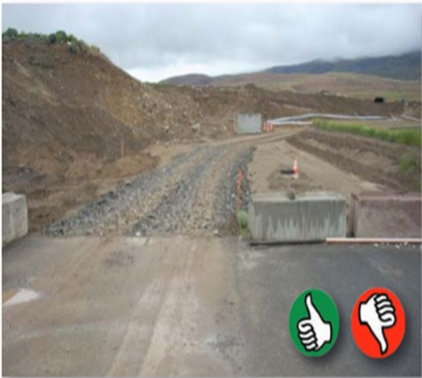
Good installation of a construction entrance, but sediment is still being tracked off-site. Add more rock or make entrance longer. (Source: Douglas County)
